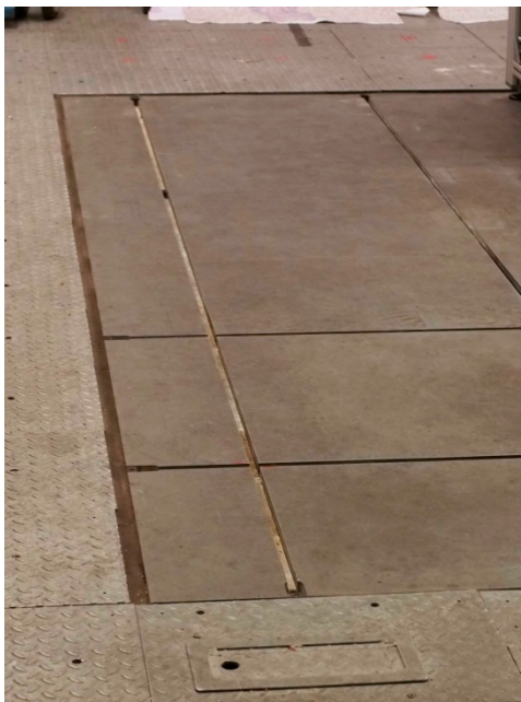
Figure 4-9. Gaps between the plates available for communication between the main volume of the facility and the underground room.
